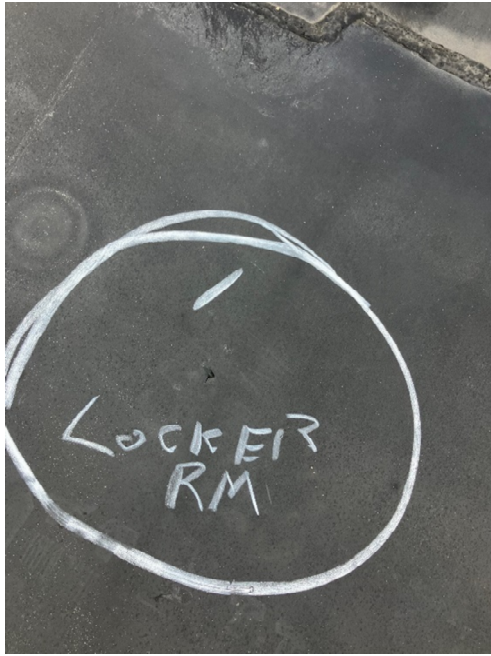
EPDM Roof Membrane Punctures
