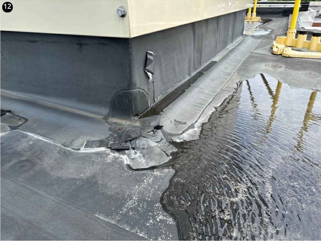
Multiple flashing issues around large units and some ponding water that will need to be corrected
