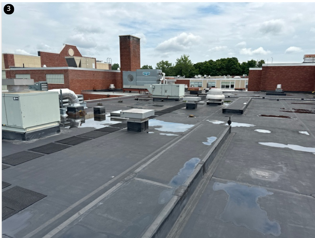
3 View of roof nine and some ponding water areas
