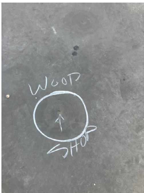
Exterior EPDM Roof Puncture
