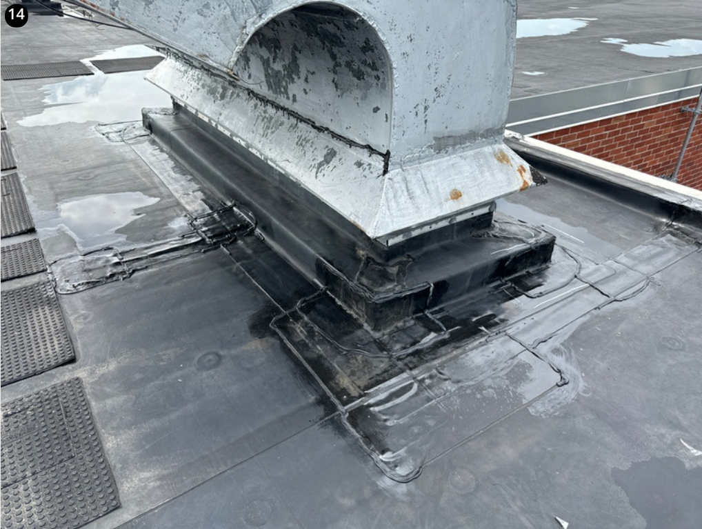
This old vent has clearly had quite a few issues and has been repaired multiple times
