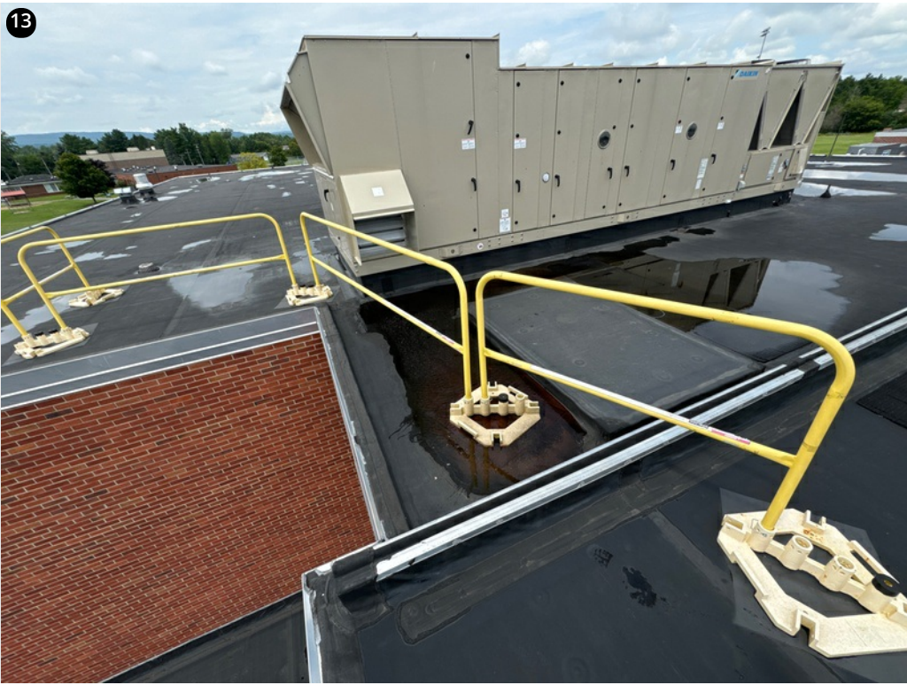
This is a pretty long run to the drain a simple spout scupper may help fix this issue pretty quickly. This is on the edge of roof 8 and 18
