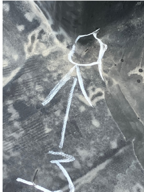
Roof Curb Flashing Failure
