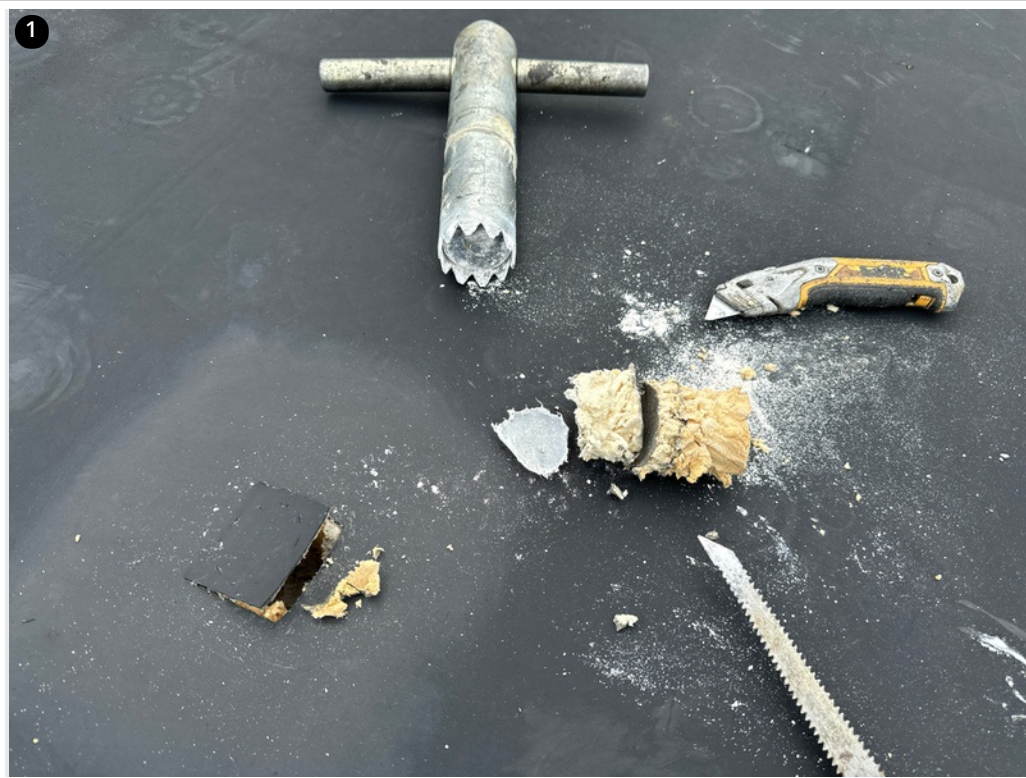
View of roof core on roof number nine totally dry with approximately 4 inches of insulation and a poly vapor barrier against what seems to be a gyp or lightweight concrete deck surface
