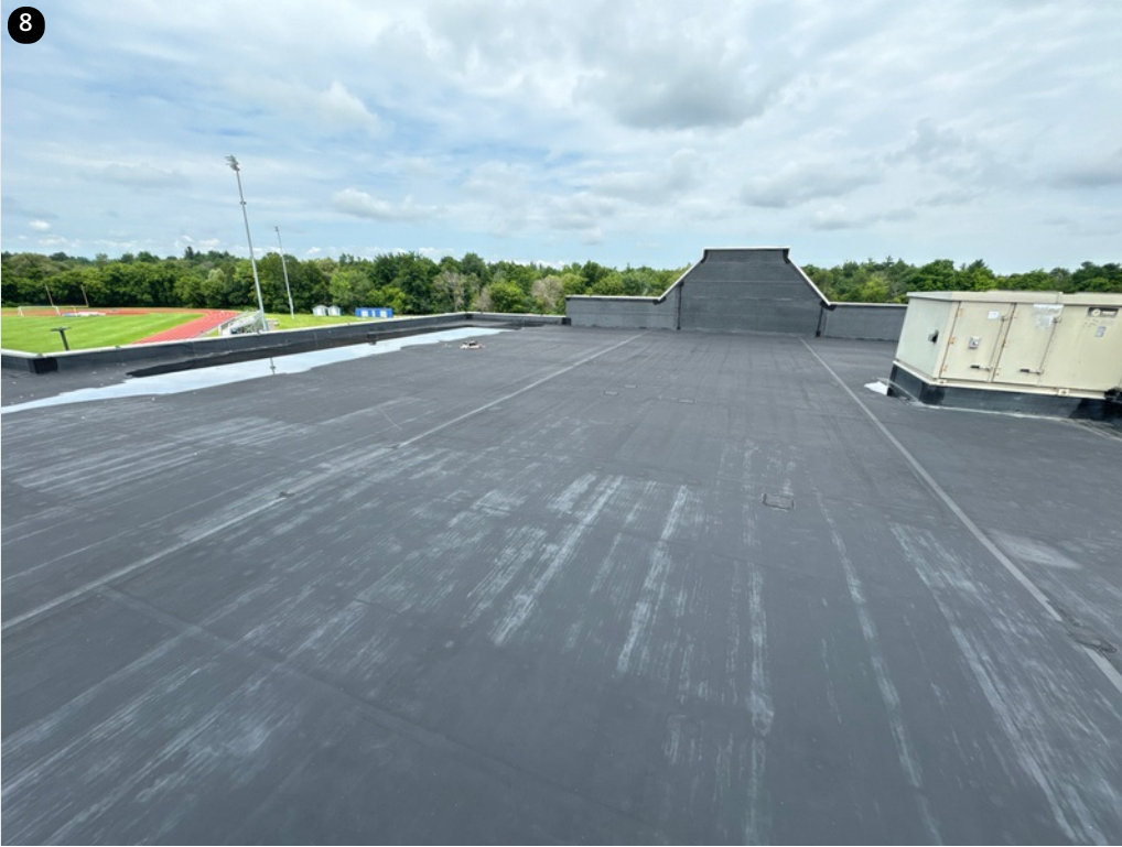
Overall view of roof section 12 there is no sump or proper taper around the drain areas
