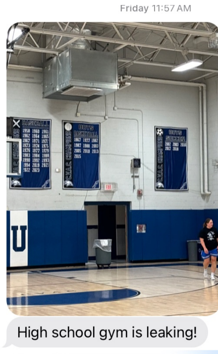
High school Gym. Trash can to catch roof leak water
