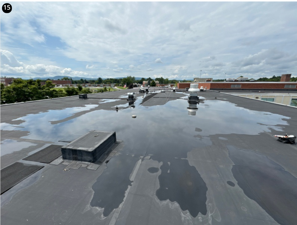
View of large ponding water area on roof number 26 the drain is clogged and needs to be kept clean
