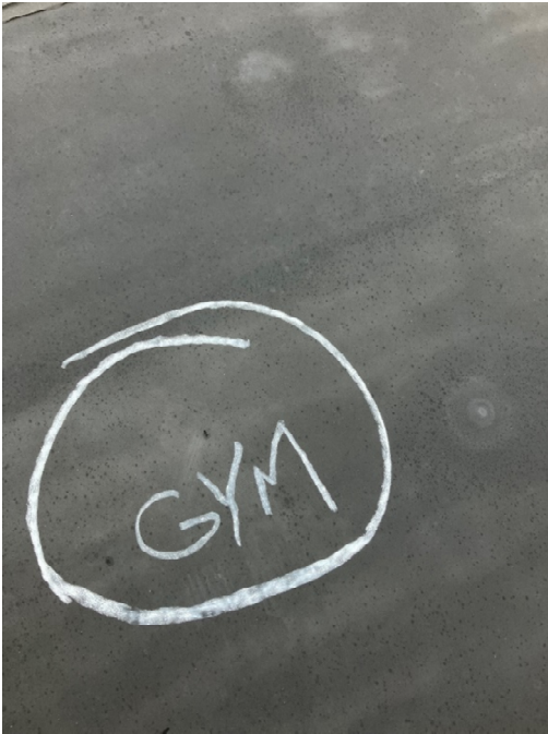
EPDM Roof Membrane Punctures
