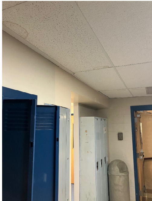
HS Roof 26 – Stained tiles
