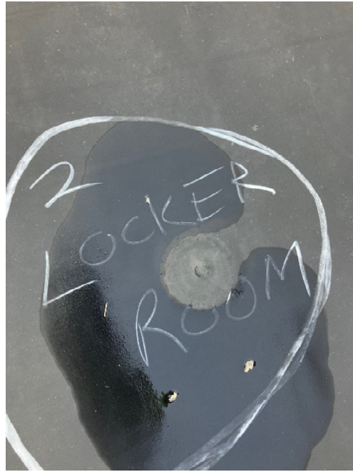
EPDM Roof Membrane Punctures
