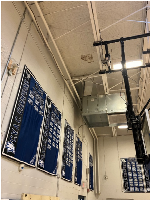
HS Roof 18 – Stained Ceiling Tile
