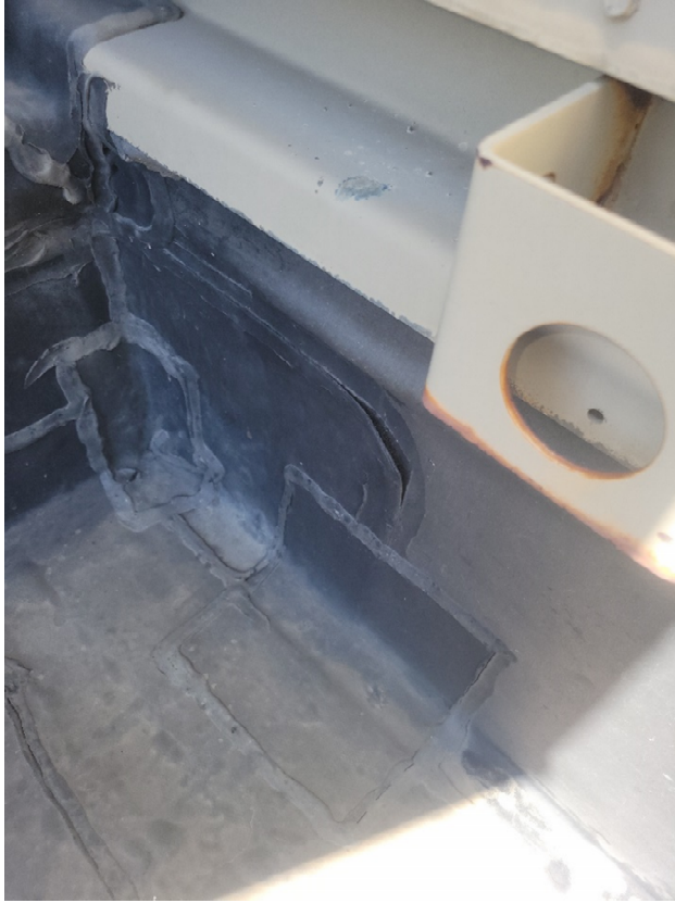
MS Gym Roof 1 flashing failure
