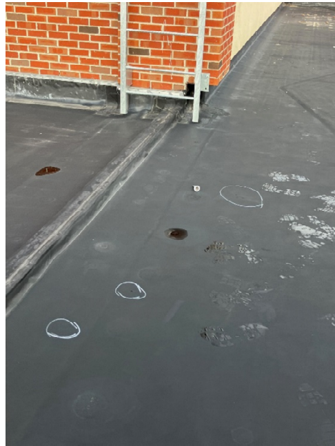
EPDM Roof Membrane Punctures
