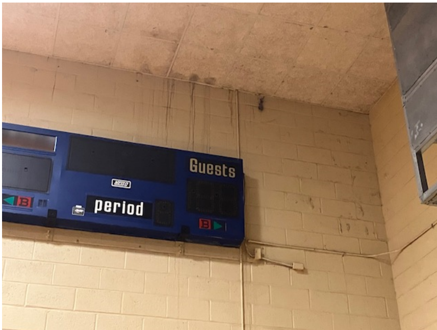
Intermediate Gym roof 19 Roof Leaks
