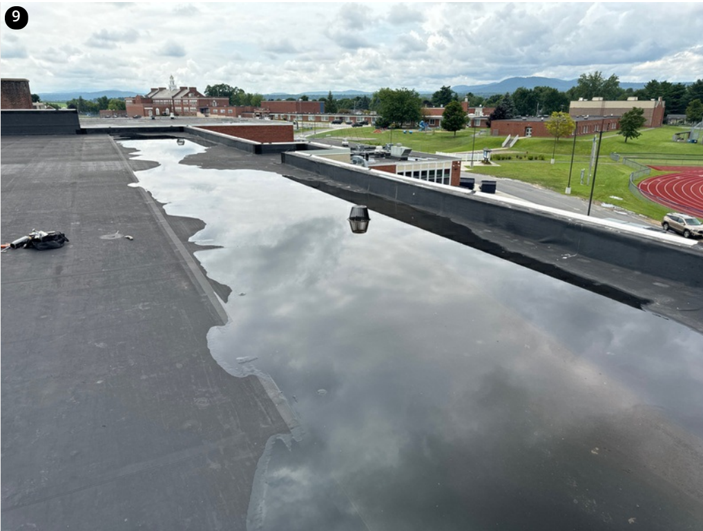
Ponding water holding on the edges of the roof
